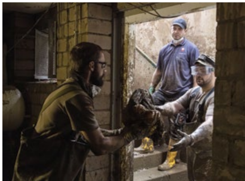
Ahrweiler: Caritas employees organised the neighbourhood scheme urgently required immediately after the flooding.
